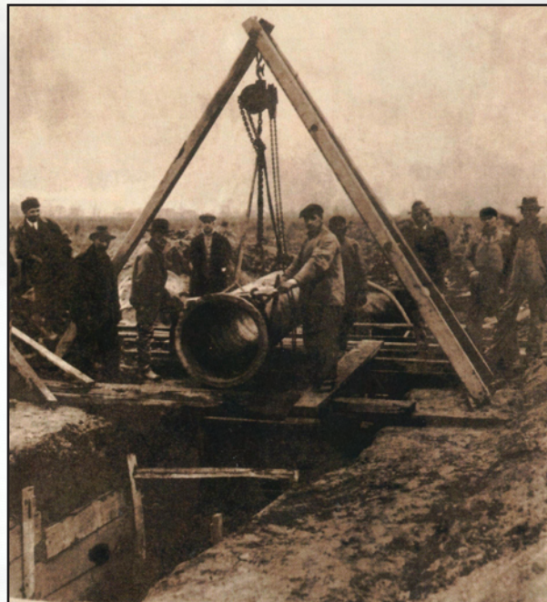
This postcard is an example of the sewers that were installed in the late 19th century. Many of these sewer lines are still being used today. In Postcards from the Past, Vol. 1 by David L. Newman.
